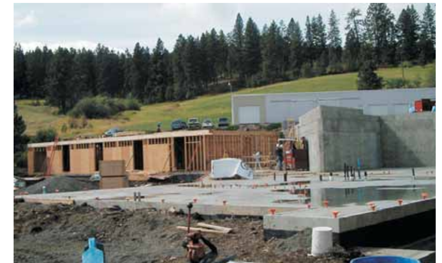
Walls are going up on the residential wing. The conference wing is in the foreground.
