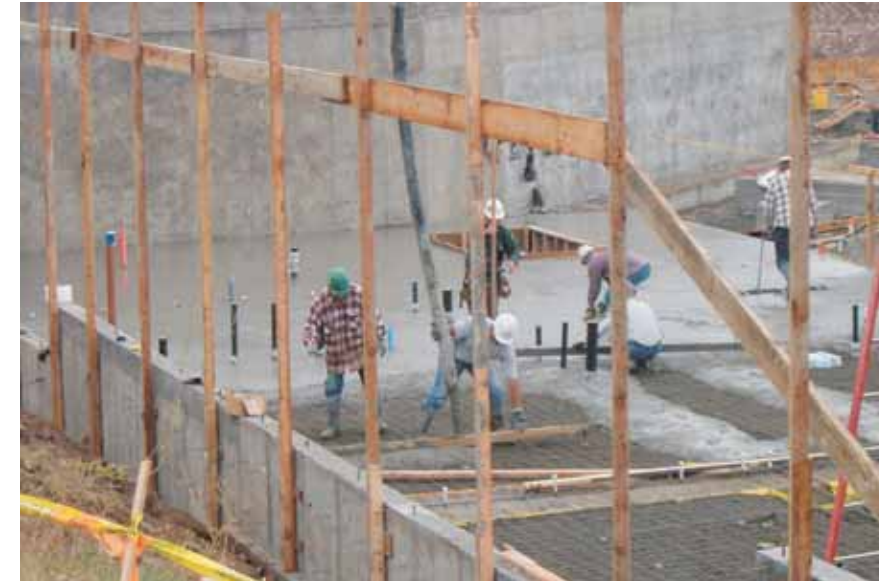
Construction workers pour the cement floor in the residential wing on cold and rain-threatened day.
